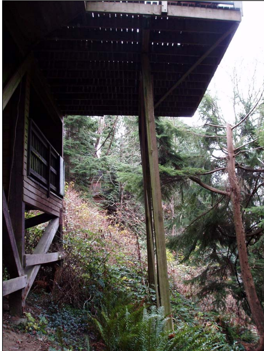
Plate 2: Note the displacement of the post supporting the deck on this structure (thought to be at 2101 Westview Drive). The crest of the ravine is located next to the base of these posts. The BC Hydro RoW is in the background of the picture.
