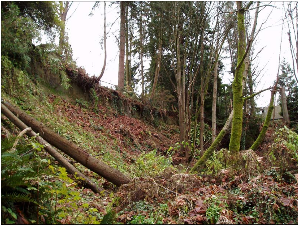
Plate 4: Looking at the scarp in a southeasterly direction. Note the debris pile in the foreground of the picture from the recent landslide at the north end of the scarp. The adjacent properties are 1931 to 1945 Westview Drive.
